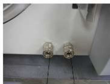
Used water manual draining hole
